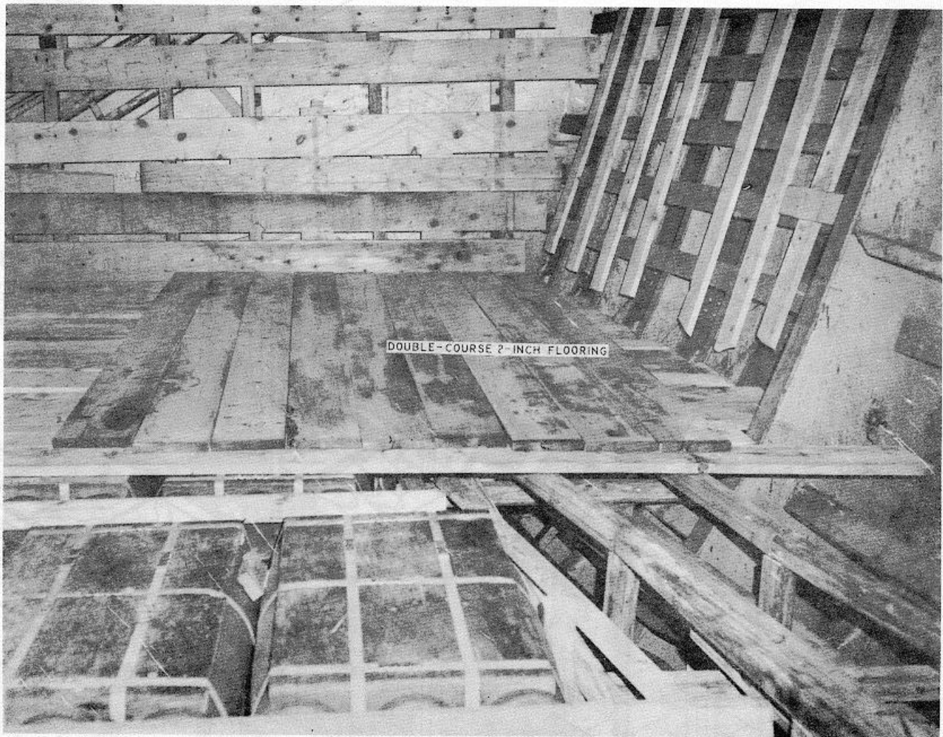
Figure 9-49. Completion of flooring prior to stowage of additional tiers of bombs (hull blocking technique).
